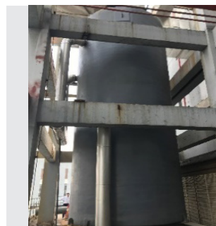
Direct contact type (suitable for 70t gas boiler)(Φ4m*14m)
