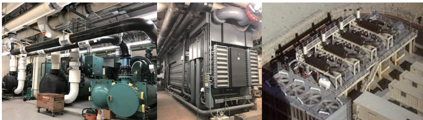
Morongo Casino Mechanical Room 摩洛哥赌场机房
