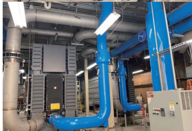
BYU's Mechanical Room 杨百翰大学机房
