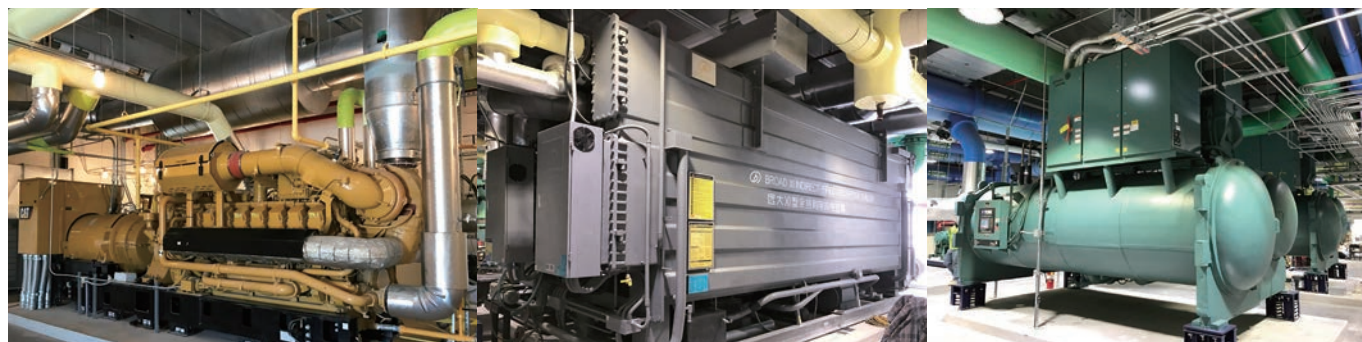
Mechanical Room of Pinellas County Jail 皮涅拉斯县监狱机房
