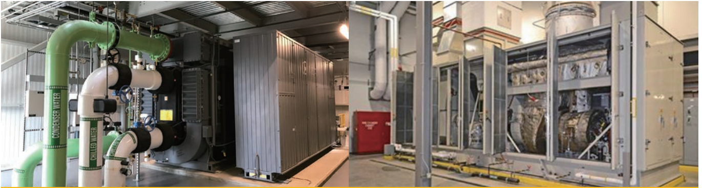
Baystate Medical Center Mechanical Room 贝斯泰医学中心机房
