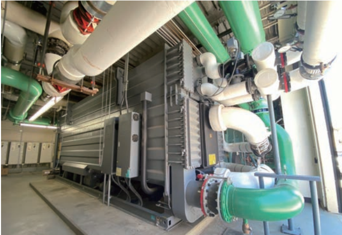
Morongo Casino Mechanical Room 摩洛哥根赌场机房
