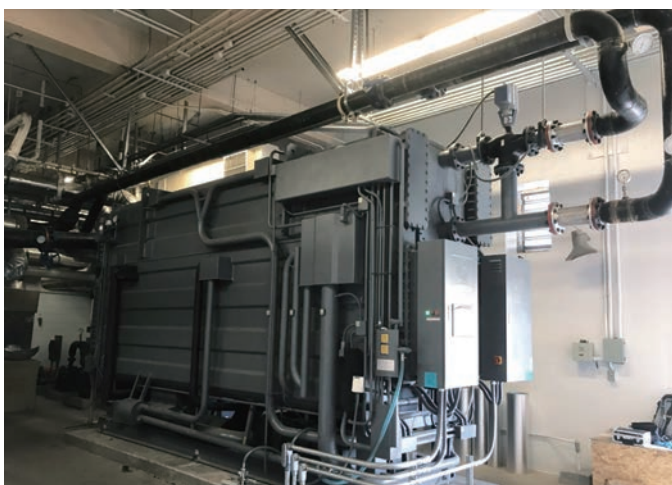
CVWRF Mechanical Room 制冷机房
