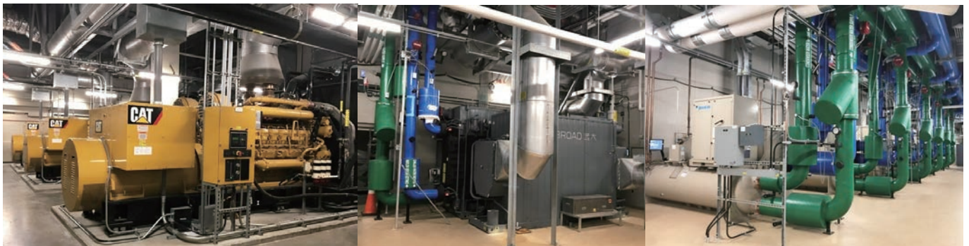
MGM National Harbor Mechanical Room 米高梅国家港口机房
